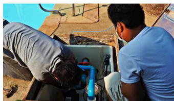
INITIAL INSPECTION OF EQUIPMENT AT SITE
